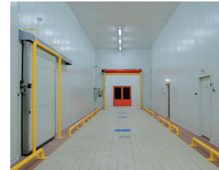
Cold Storage Warehouse
